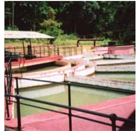
Matale Water Treatment works
